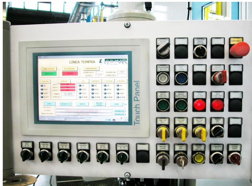
Displayed details on one production line's work substations. Each substation is equipped with an operator control unit and HMI touch panel based on Movicon for Windows CE, connected through LAN Ethernet with the Movicon Supervisor.
